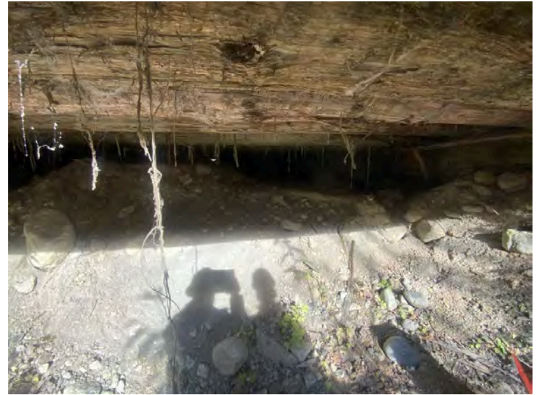
Accumulation under bridge
